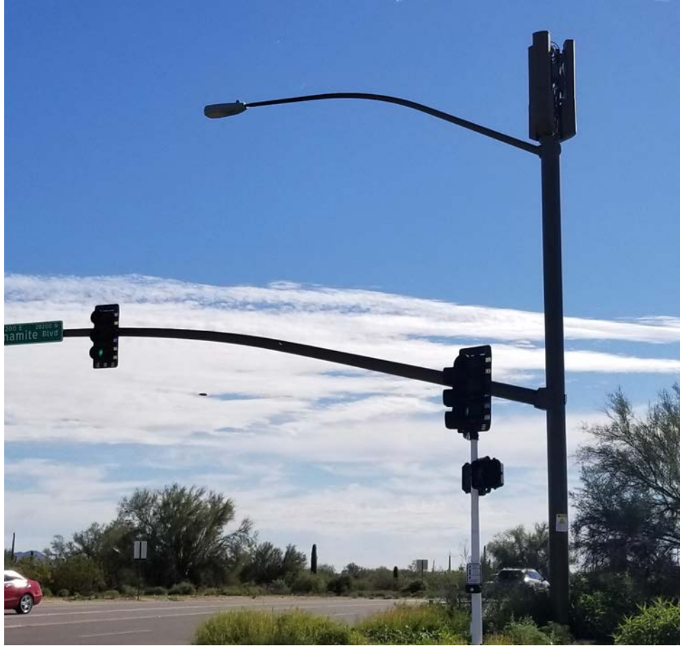
Small Cell Installation Nationwide
