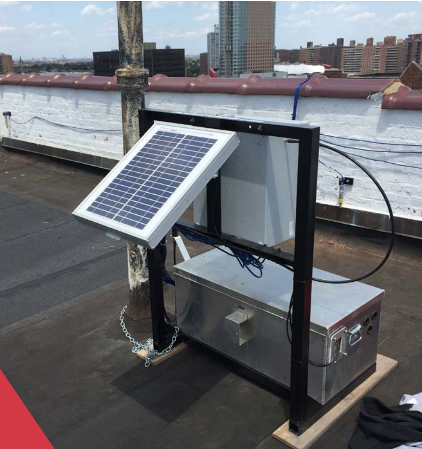
NYCDDC Tilt Monitoring, New York, NY
